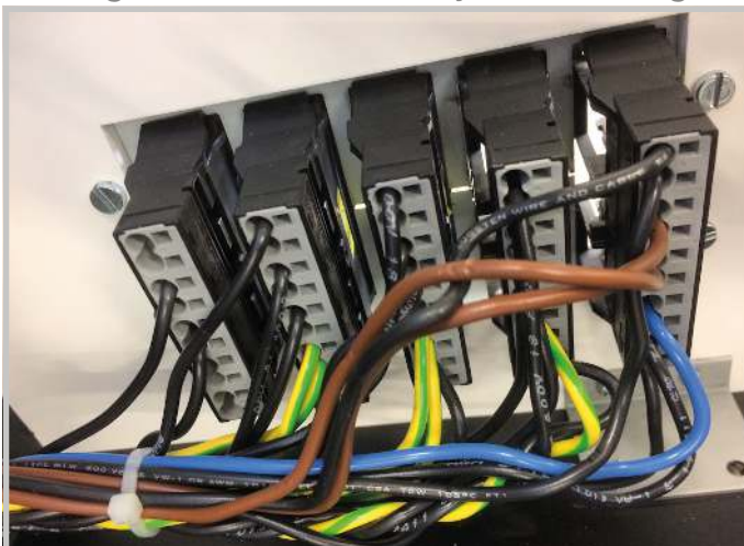
4.7 Missing cable ties and messy cable routing
